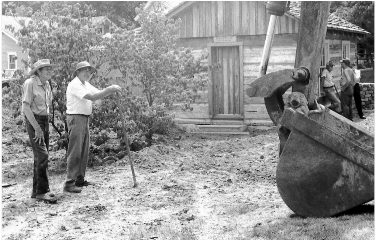
Coach Dean and Roy Robertson oversee efforts to construct the Pioneer Village. (The JHC, Circa 1979)
